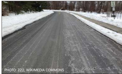
Roadway With Salt Residue
