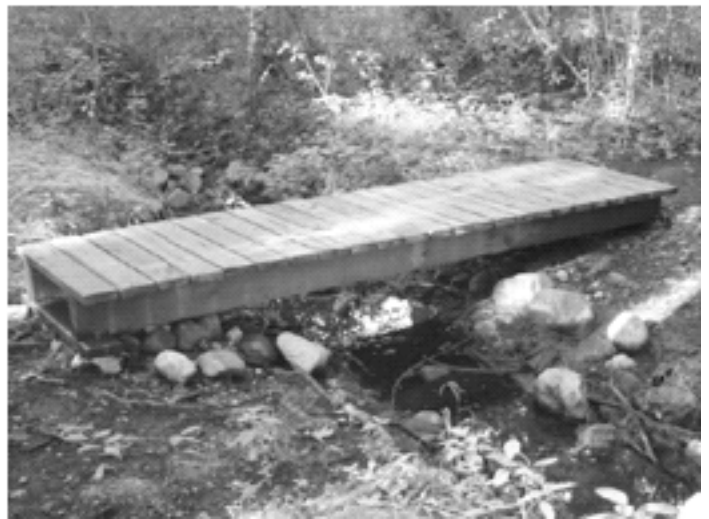
One of the two new bridges constructed at the Flowed Meadow Conservation Area (photo by Matthew Gray)
