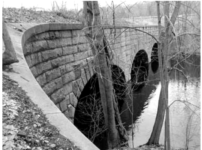
Bridge carrying Cochituate Aqueduct from Wellesley to Newton across the Charles River near Routes 16 and 128. (Photo courtesy of Middlesex Canal Association Website)
