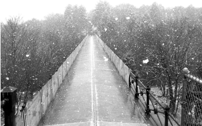
Temporary snow fence installed along the deteriorating iron railing atop Echo Bridge. (photo by Bill Hagar)
