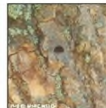
Damage Exit Hole
