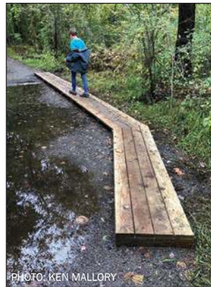
New wooden walkways installed by Alex Rivero and Scout Troop 9 now help park visitors negotiate rain accumulation through Cold Spring Park.
