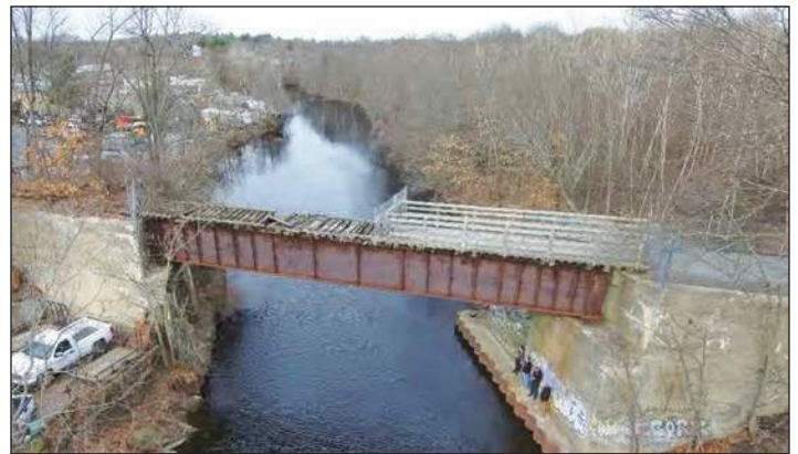
Project limits and bridge photos shown excerpted from the GPI study report
