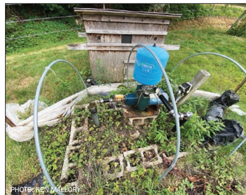
Ground water well and irrigation system at Newton Community Farm.
