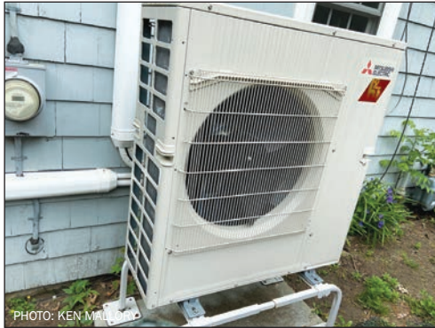
Mini split heat pump used for home heating during winter and cooling during summer.
