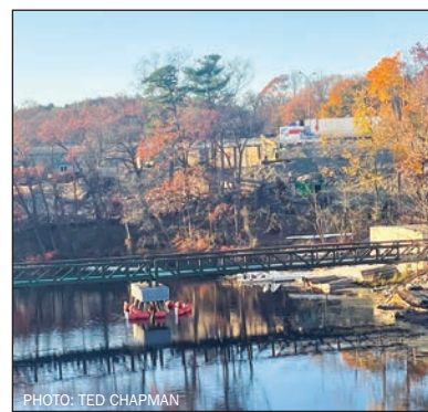
Stoller Bridge/Pigeon Hill Rd.: The Recreation Road/Stoller Boathouse Bridge under construction with the I-90 Pigeon Hill Trail construction in the background.
