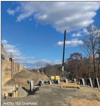
Pigeon Hill I-90 east: Looking east from Pigeon Hill the steel foundation for the abutment under construction; the Pigeon Hill Trail will run downhill on a shelf created to the right (river side) of the new abutment.
