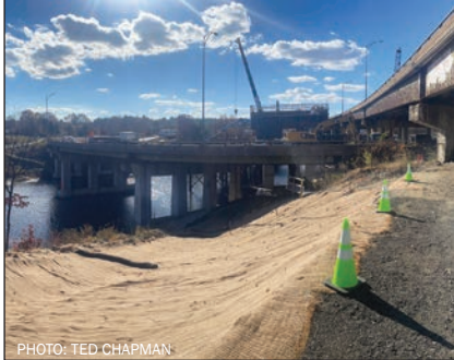
Pigeon Hill I-90 West: Looking west from Pigeon Hill, the new piers for I-90 east roadway are rising across the Charles River 40 feet south of I-90s current location. The Pigeon Hill Trail will run under this roadway.
